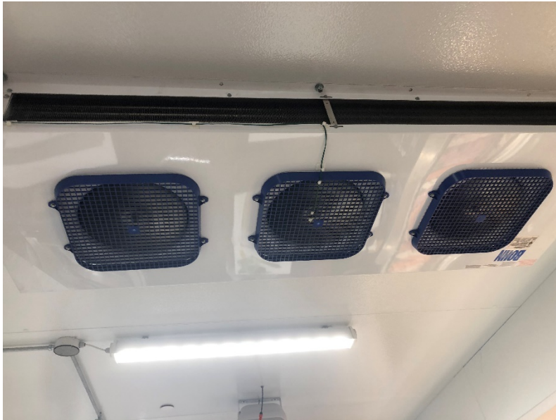
1. Photo of the current fan in the space
