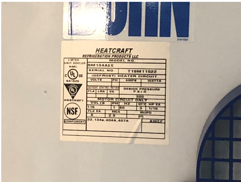
2. Closeup photo of the nameplate of the current fan
